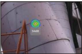
Vacuum Leak on a Cement Kiln
