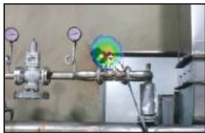
Compressed Air Leak on an Isolation Valve
